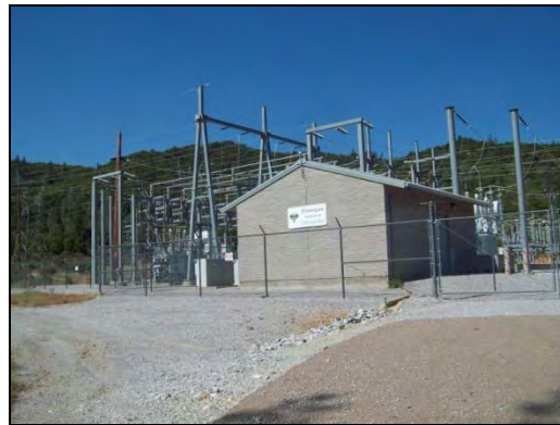
City of Shasta Lake Substation
