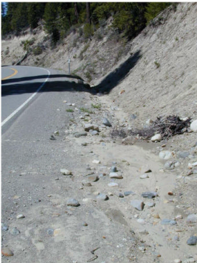
Eroding cutslope and inside ditch delivering water and sediment to a small stream channel.
