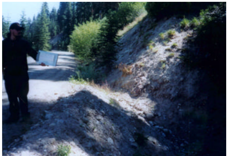
Inside ditch draining directly to a stream.
