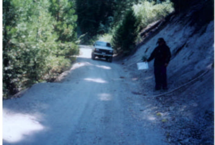
Cutbank and road surface eroding next to a stream channel.
