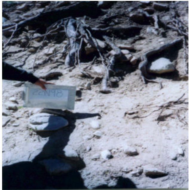
Erosion void measured by root exposure.
