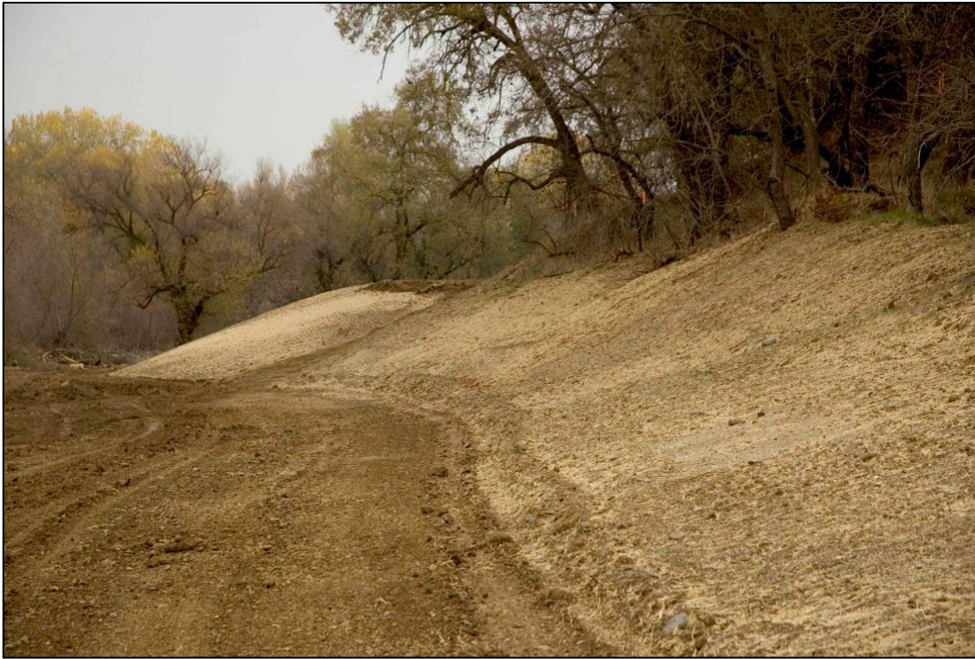
Stabilized and seeded (native creeping wildrye) streambank along south bank of Putah Creek at confluence with Dry Creek, in December 2005, following channel realignment in September to protect Putah Creek Road (see Exhibit 4-3b.(h) showing failing bank prior to realignment).
