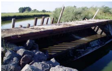
Pit River Dam. Water impoundment structure along Pit River used to raise water levels in the river during the summer to irrigate pastures and crops.
