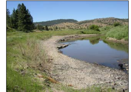
Bank stabilization at Shaw Ranch using rock vanes, bank reshaping, and willow planting.
