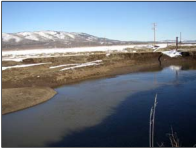
Channel erosion, Pit River near Lookout.
