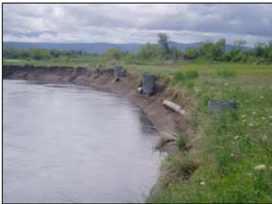
Bacigalupi Ranch Erosion has exposed the water conveyance system.
