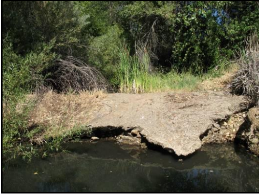
Outflow Obstruction near mouth of Rock Creek.
