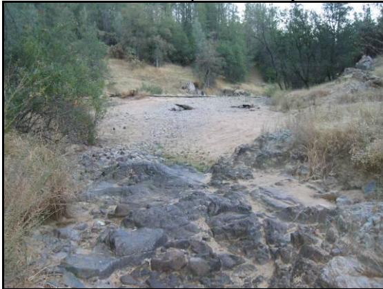
Sediment Buildup at Swasey Dam.
