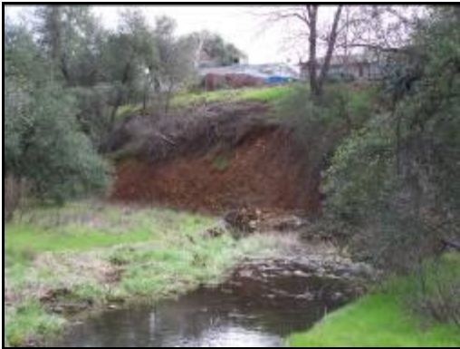
Bank eroding below homes
