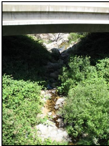
Channel Encroachment near bridge on Middle Creek
